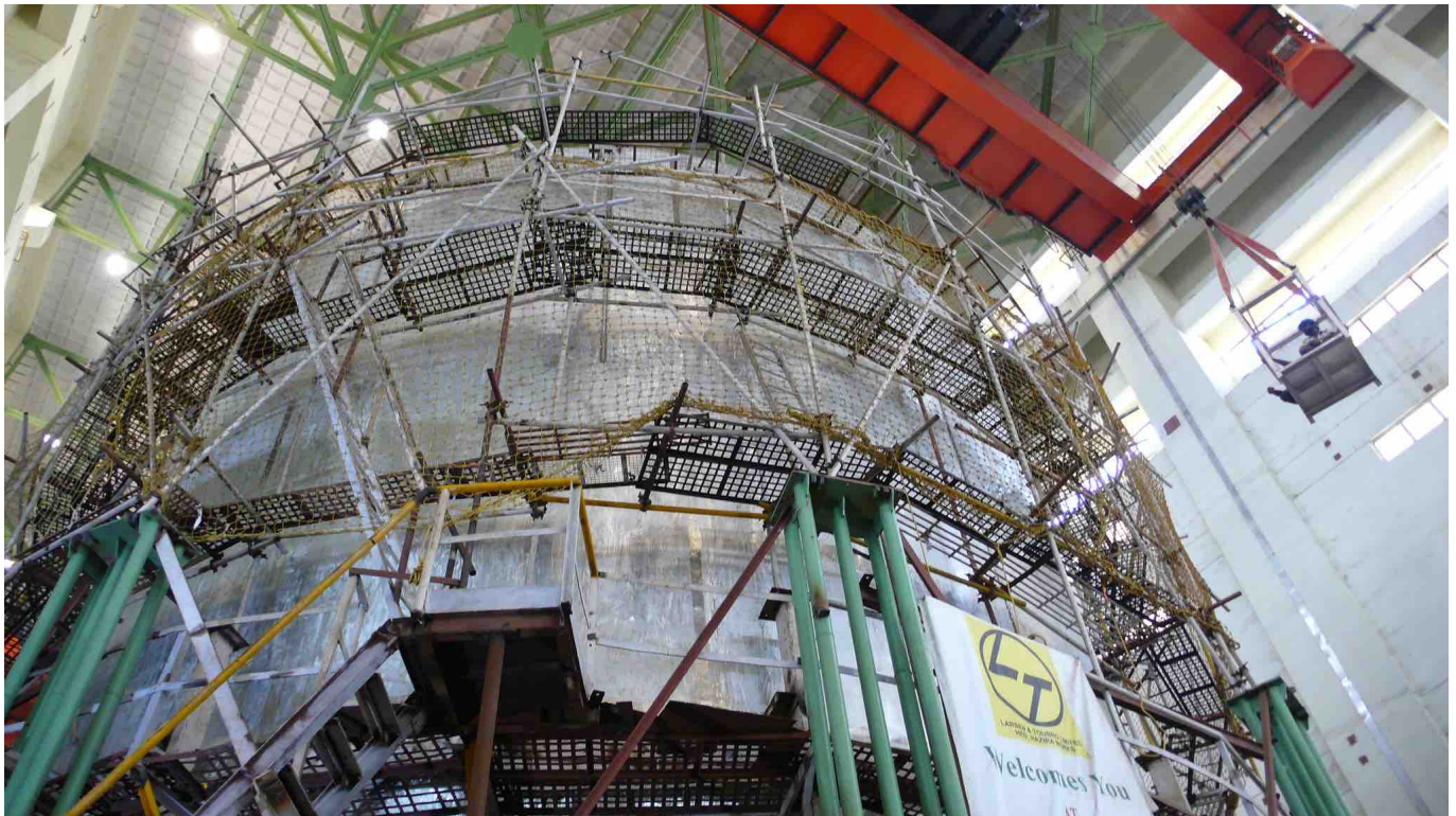
The Fast-Breeder Nuclear Reactor under construction at the Kalpakkam Nuclear Complex (2013) | Petr Pavlicek/IAEA
